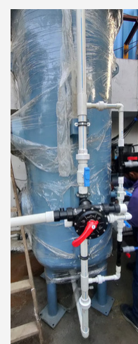
20 M3/Hr MB Plant at Chakan
