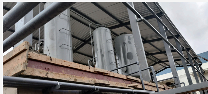
5M3/Hr Water Softener at Jejuri
