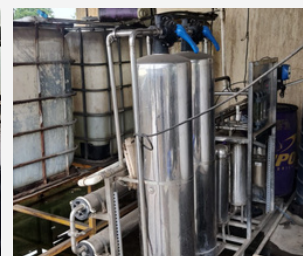
500 & 250 LPH RO at Pune
