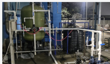
25M3/Hr Water Softener at Kolkata
